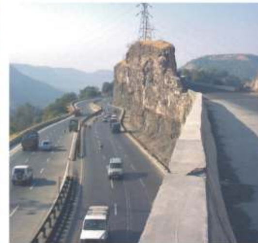
Landslide and Rockfall Site on Mumbai-Pune Expressway–CSIR provided remedial measures to prevent rockfalls in this region.
