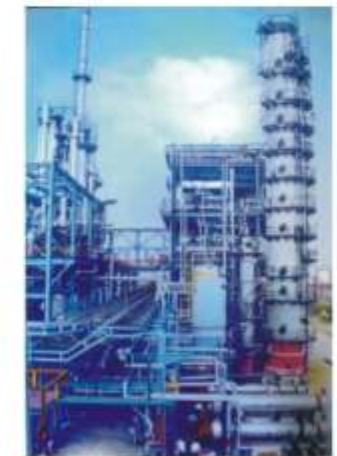
NMP Lube Extraction Plant
