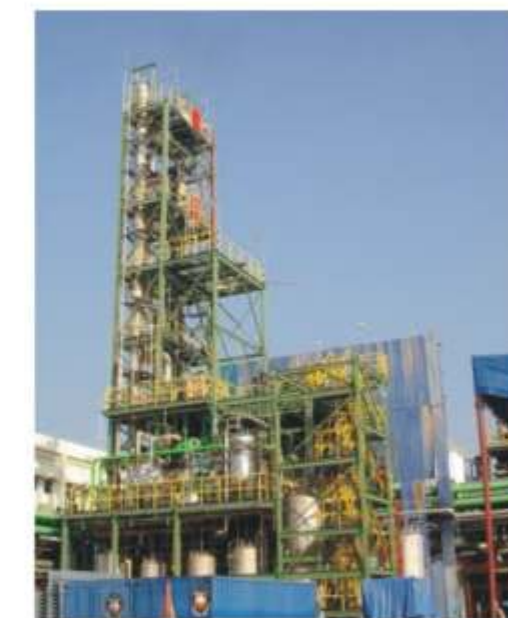
View of 3000 tpa epichlorohydrin plant – First plant of its kind in the world. Commissioned in Thailand
