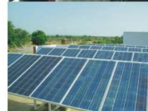
First Community Solar-based RO plant of 700 litres per hour capacity installed in Sambhar Lake of area of Rajasthan
