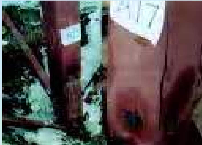
View of crack in column
