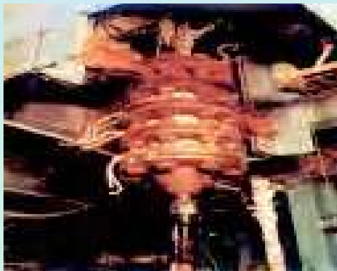
Soaker Reactor With Internals
