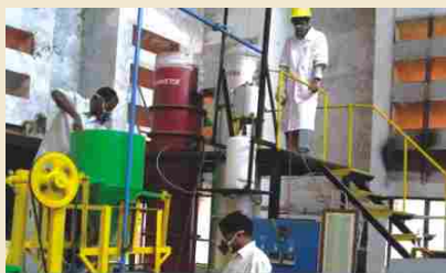
Fig. 1.42: Prototype of entrained flow biomass gasifier system
