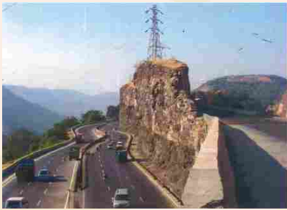
Fig. 1.34: Landslide and rockfall site on Mumbai-Pune expressway
