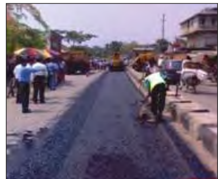
Fig: 1.51b Laying of cold SDBC in Guwahati as demo for Assam PWD
