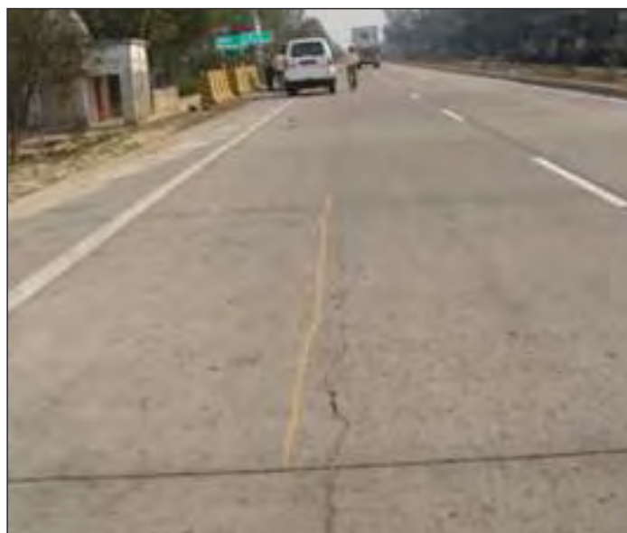
Fig: 1.48 Longitudinal crack in outer lane
