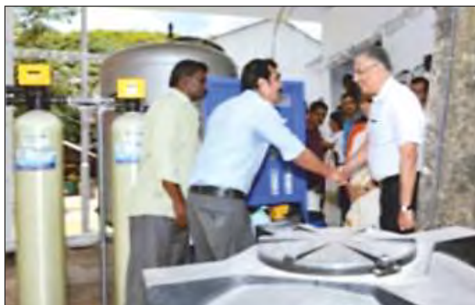
Fig: 1.97 Dr. Suresh Das, Director, CSIR-NIIST, inaugurating the Drinking Water Plant
