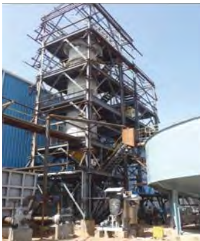
Fig: 1.62 Flotation Column (2.5m dia) erection work in progress at Andhra Baryte Corporation Pvt Ltd, Mangampeta, A.P. for the beneficiation of low grade barytes
