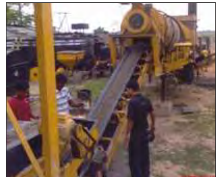
Fig.: 1.51a Production of emulsion based cold mix by Hot Mix Plant (Switching Off Heating Arrangement) in Guwahati
