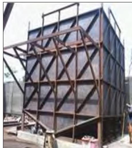
Fig: 1.40 Glimpse of FICCO Plant
