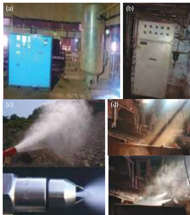
Fig. 7.24: Dry fog dust suppression system installed in Donimalai Iron Ore Mine of NMDC Limited:
