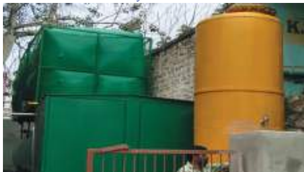
Fig. 6.2.4: Full scale biogas plant for the treatment of food waste at Kurnool, AP
