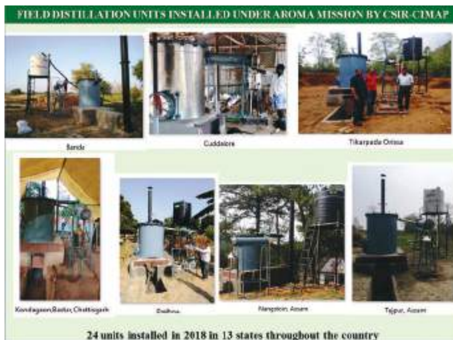
Fig. 6.4.3: 24 Units installed in 2018 in 13 states throughout the country
