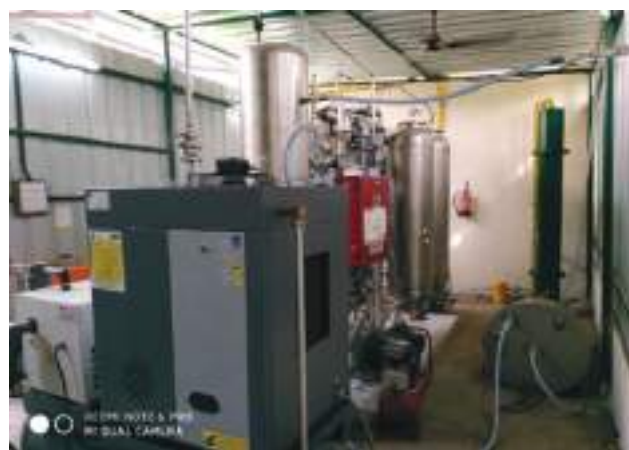
Fig. 7.9: CSIR-IIP's Biogas Up-gradation Plant Installed at Pune Municipal Corporation's Katraj Site
