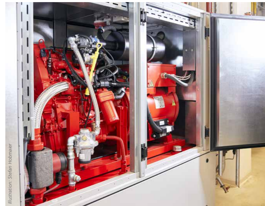
Cogeneration unit for power-heat coupling: an integral part of energy systems.
