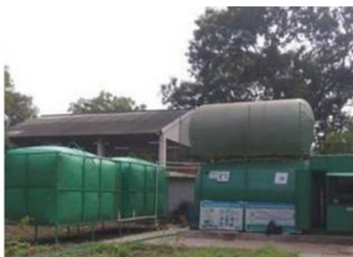
Anaerobic Gas lift Reactor
