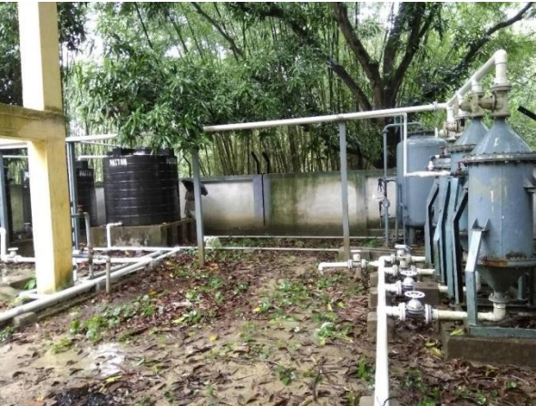
10m 3 /hour Iron and Arsenic removal plant by CSIR-CGCRl
