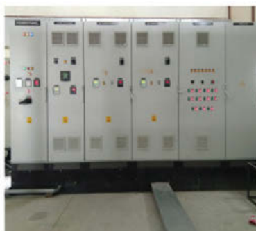
Power panel for Industrial grade Autoclave
