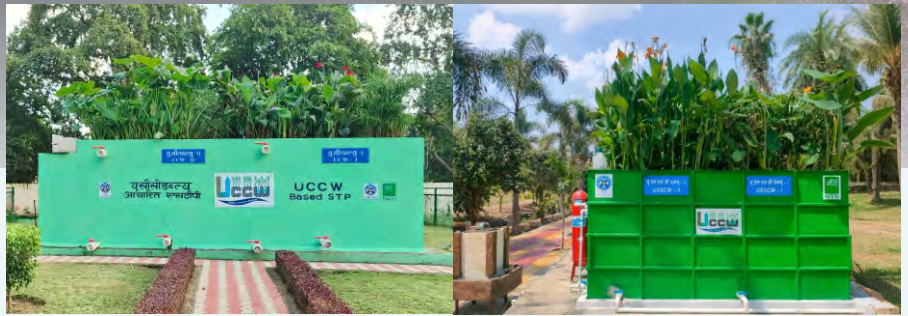
15 KLD packaged modular UCCW-based STP, installed at CSIR-NEERI, Nagpur (Left); 25 KLD institutional plant at CSIR-CSIO, Chandigarh (right)
