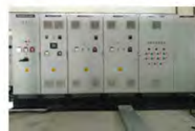
Power panel for Industrial grade Autoclave
