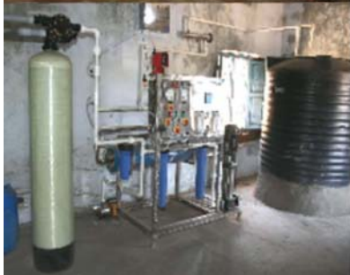
Defluoridation plants at Allapur, Nerimetta, Rachakonda & Gaggalapally
